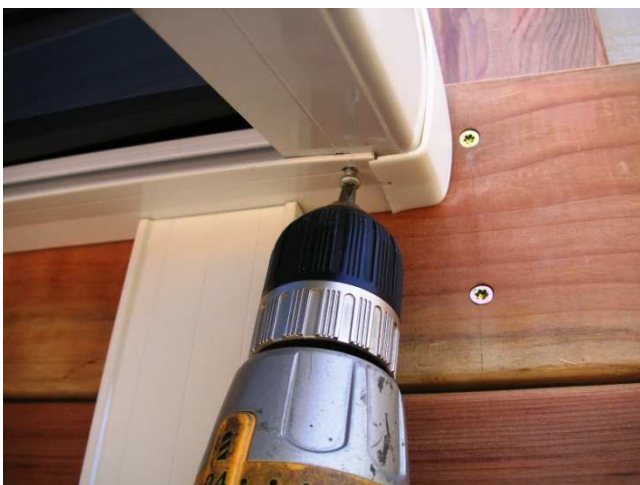
20. Secure the middle rafter(s) and the right edge rafter with self-tapping screws in the back and front.
