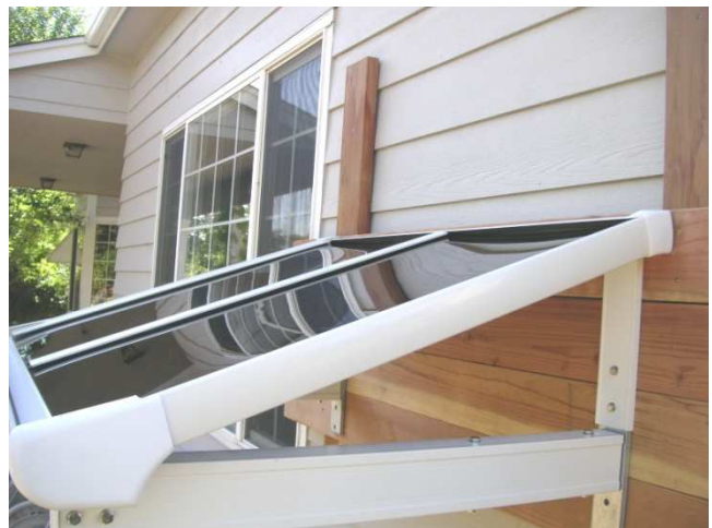
19. Apply caulk along the inside edge of the gutter (see Step 12). Install the right edge rafter with front and back caps.
