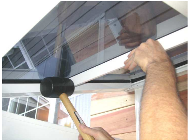
23. Install polycarbonate sheet middle supports and adjust their positions using a mallet.
