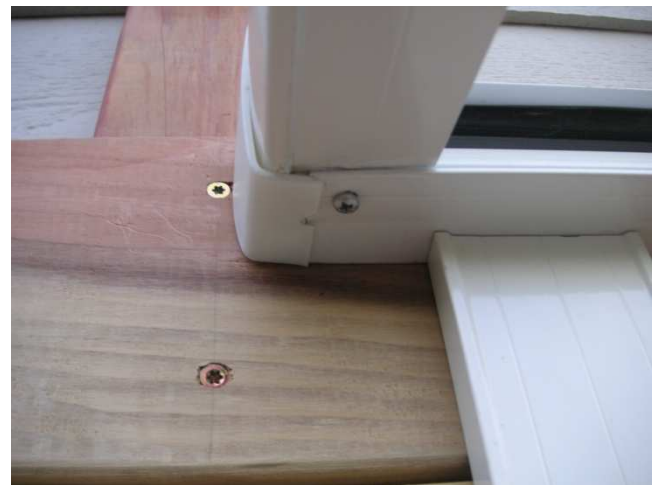
15. Secure the left edge rafter with self-tapping screws in the back and front.
