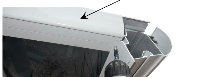
15. Install the edge rafters and secure them to the header and the gutter with self-tapping screws.
