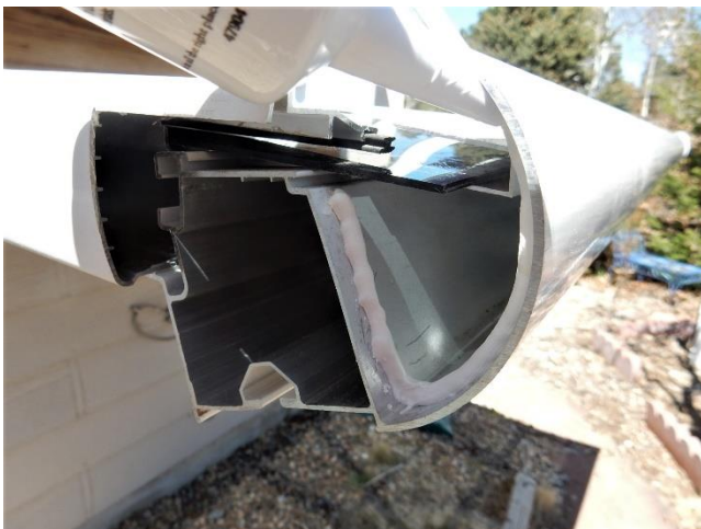
16. Apply caulk along the inside edge of the gutter on both sides to prevent water leakage through the gutter and cap connection.
