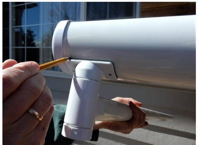
23. Mark the water receptacle position on the left or right side of the gutter, with an appropriate drain pipe slope toward the wall.
